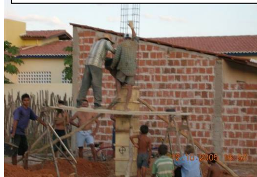
Ps Esteves and crew working on concrete pillars for the new hall at Gadelha
