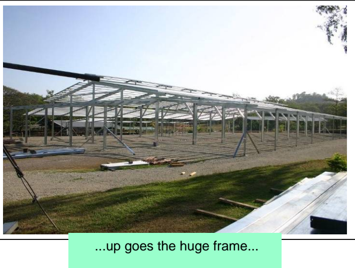
After months of planning and the lengthy approvals process the massive earthworks begin
